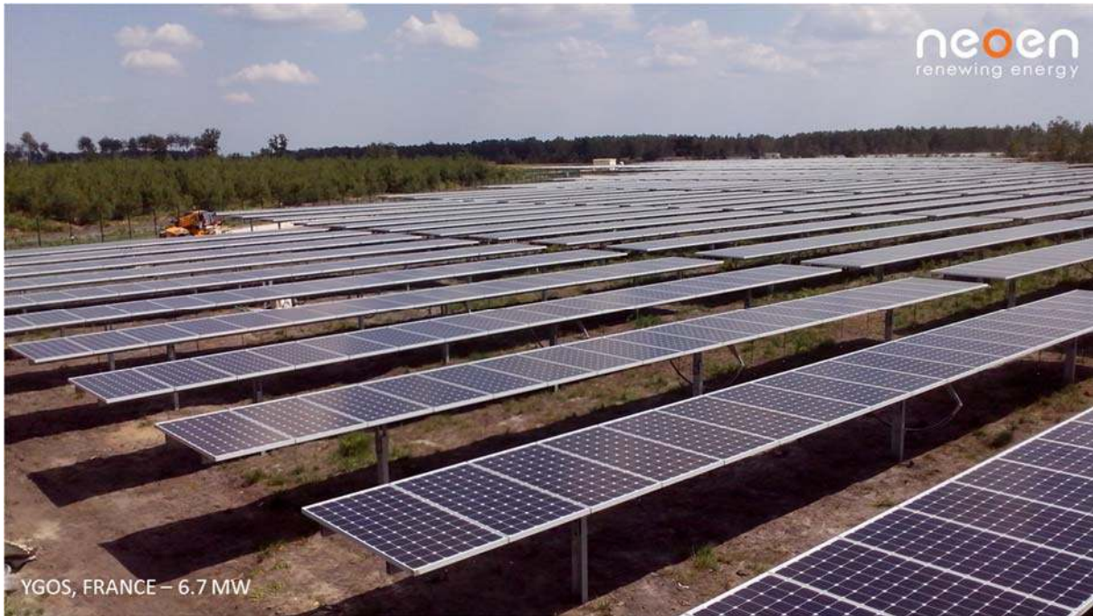
Figure 2-3 Example of single-axis tracking systems with multicrystalline modules
