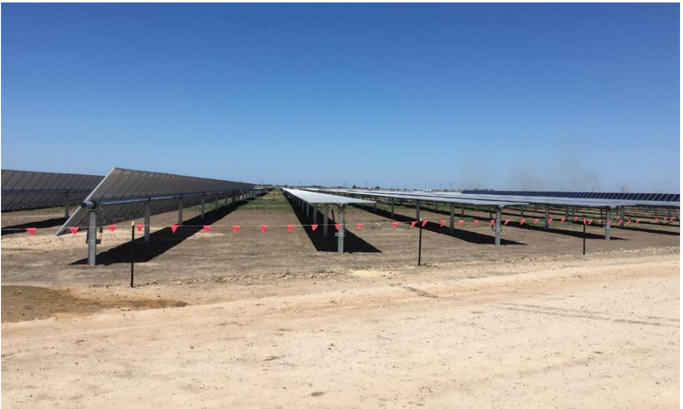
Solar Tracker Testing
